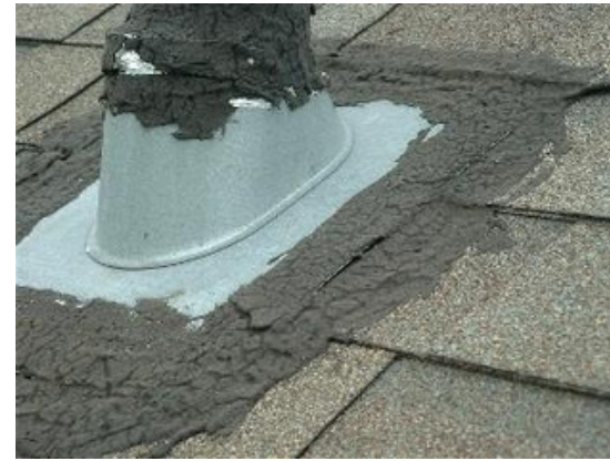
Below: This galvanized flashing has been installed improperly. The upper part of it should be under the shingles, and the roofing tar is a further sign of a poor repair.
