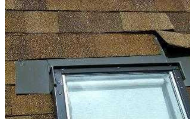
Below: The top of this flashing is not tucked under the seam of the shingle. Water will pour right in. (Courtesy of Homegauge)
