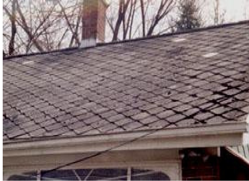
Above: diamond-pattern asbestos cement shingles
