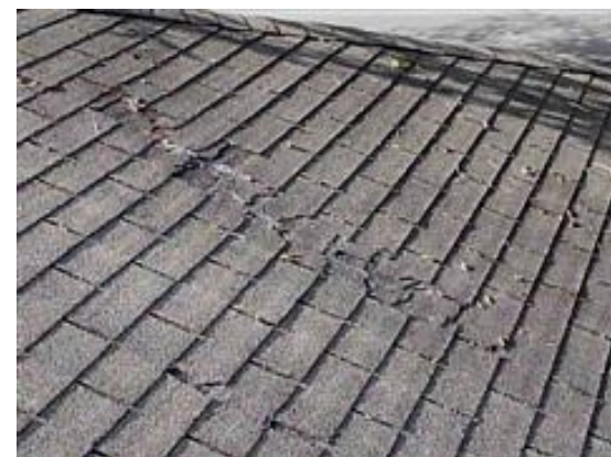
At left: another example of shingles that have been overheated by the sun and are now curling and cracking
