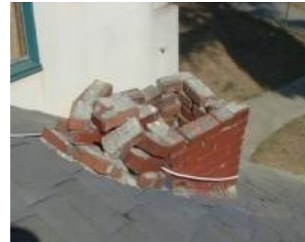
Above: This chimney has not been maintained at all, leading to a full collapse. (Courtesy of Jeff Pope)
