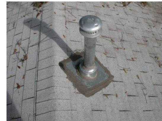
At right: This flashing has been improperly installed because the base should be underneath the shingles.
