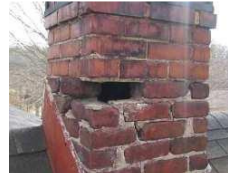
Above: A brick is missing and the mortar is spalling out.
