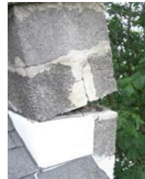
Above: A block chimney is showing such severe cracking that the top three courses are completely loose. (Courtesy of Joe Myers)
