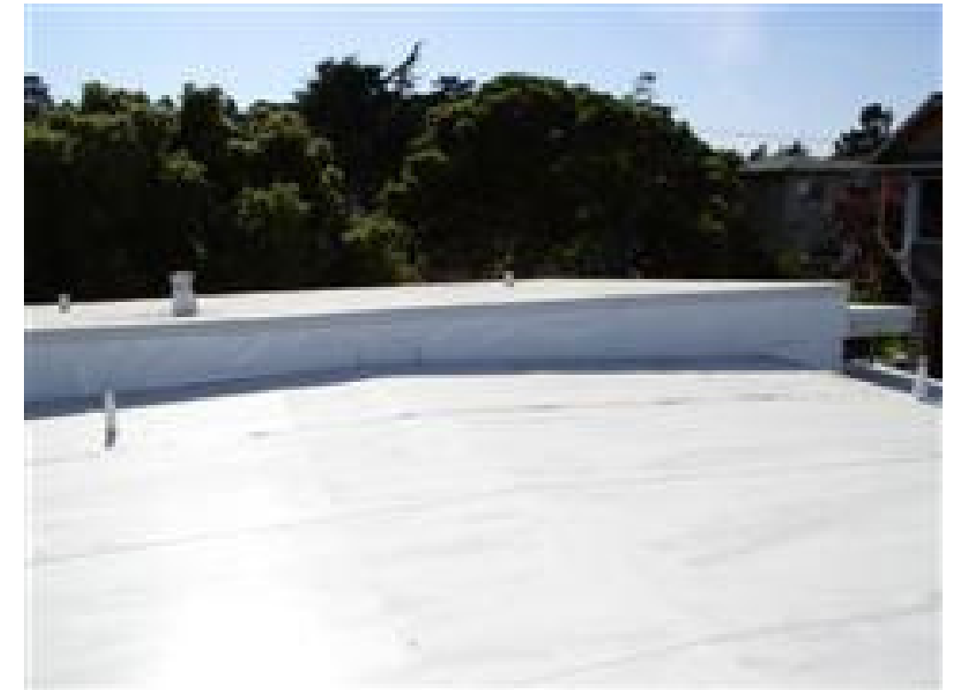
Above: This is another EPDM membrane. Notice the wrinkles between the sheets. This could easily allow water penetration. These areas need full evaluation.
