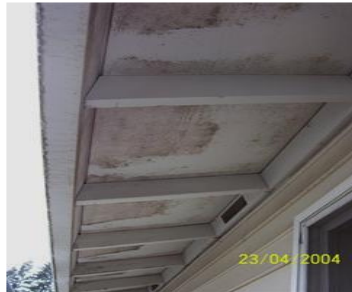
At right: open soffit with visible signs of moisture staining on the underside of the roof sheathing
