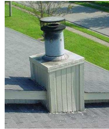
In this poorly designed chimney at left, there is no separation between the timber components and the roof, and there are a couple of dead areas which will trap moisture and promote rot.
