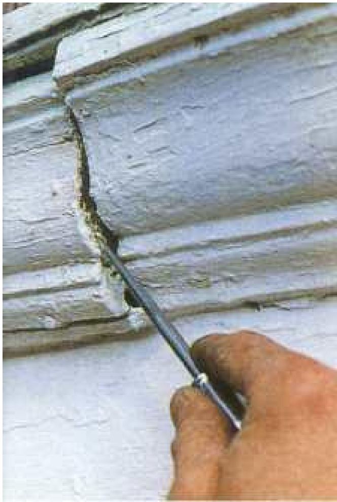
At left: Wood rot has loosened the cornice molding and is splitting around the nails.
