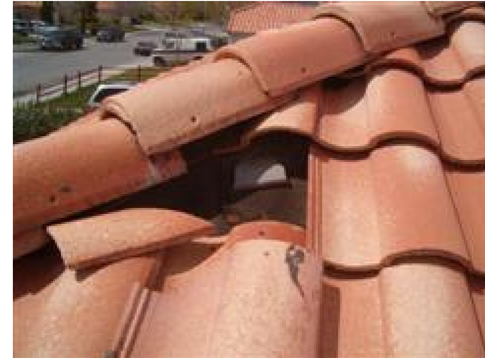
Above: impact damage on a clay tile roof showing broken and dislodged tiles
