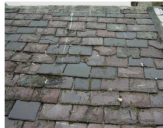
At left: an older slate installation showing many broken and dislodged tiles
