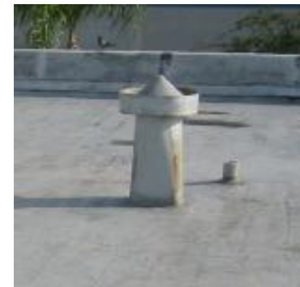
Above: This is the roof outlet for the vent system in the photo at the far left.
