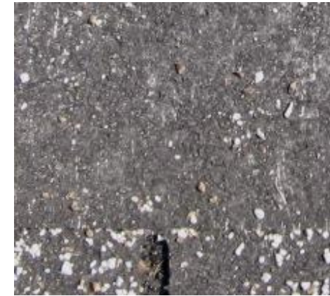
Above: an extreme close-up of a badly weathered fiberglass-based shingle whose fibers are exposed
