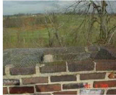
Above: This chimney has no cap or liner all. It is no longer legal to build an unlined chimney.
