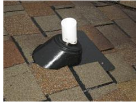
At left: This plastic vent flashing has been installed upside down. This will probably allow moisture to travel down the outside of the vent pipe.
