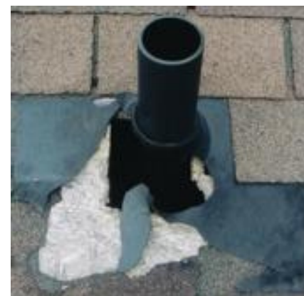
Above: This is a plastic vent flashing which was damaged by raccoons.
