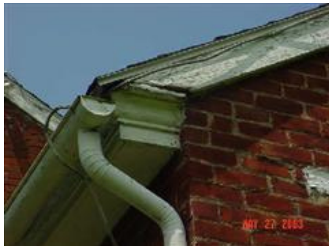
At left: rot in the lower part of the rake board; the wood has swollen and is pulling away.
