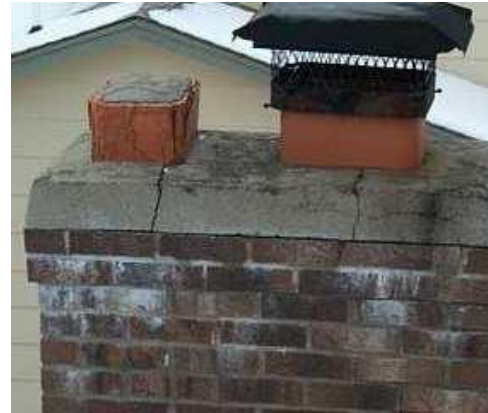
Above: The flue on the left has been sealed with concrete, and the flue on the right has a rain cap. However, the chimney cap itself is cracked and the brick work is showing signs of efflorescence.
