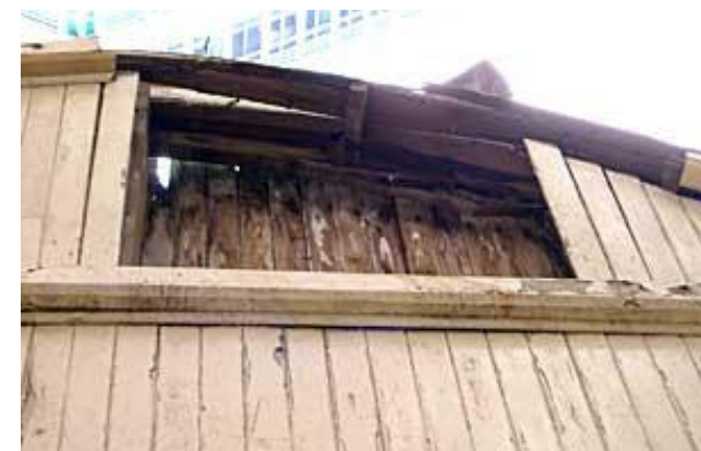
At left: older-style enclosed soffit clearly showing holes and missing boards, as well as signs of moisture in the roof sheathing
