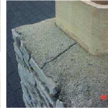
Above: cracking in the chimney cap
