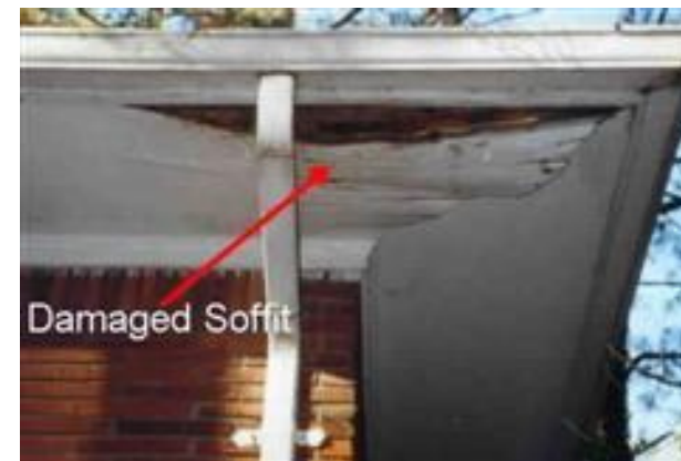
At left: standard box soffit showing signs of de-lamination due to moisture intrusion (Courtesy of Mike Rose)
