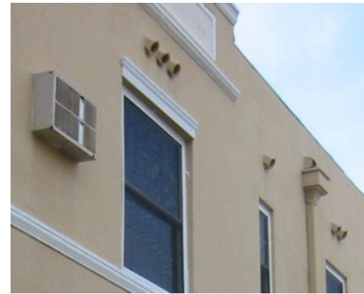
Above: The terracotta pipes shown in this wall are, in fact, part of a passive ventilation system for the flat roof above.
