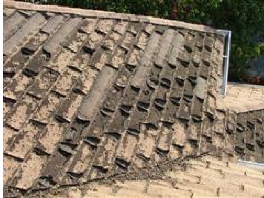
Above: an asphalt shingle roof that shows evidence of overheating, probably caused by both orientation and poor ventilation
