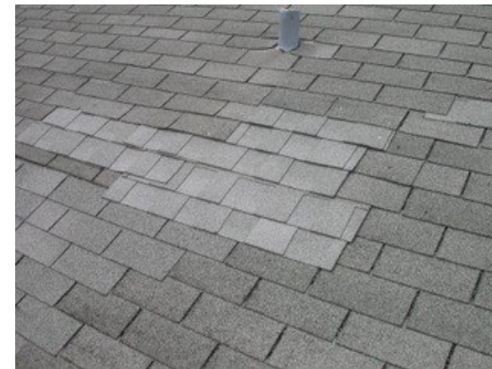
Above: Improper repairs have been made to this shingled roof.
