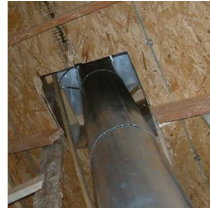
At left: This is a manufactured chimney going through the roof sheathing. The clearance on the right side is probably less than 2 inches. Also, notice how the rafter has been cut.
