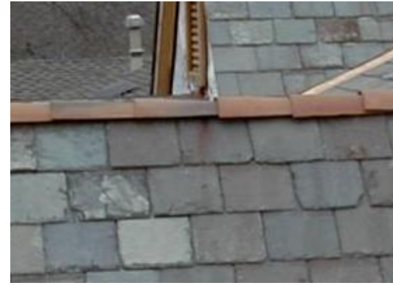
At left: an older roof; small chips at the corners of tiles are generally not of concern. Note the ridge cap, which is made of clay tile.
