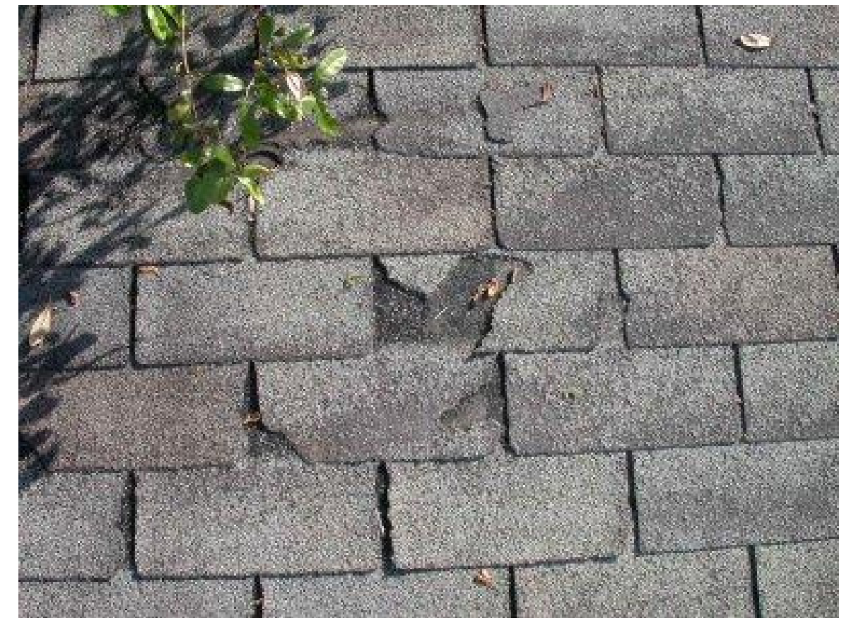
Above: a fiberglass asphalt shingle roof whose shingles became brittle over time, allowing the wind to get under them and blow them off the roof
